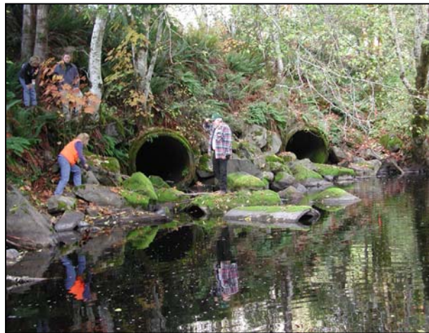
The culverts at Sherwood Creek before removal (Project 01-1237). Railroad tracks over the culverts are not visible from this perspective.
